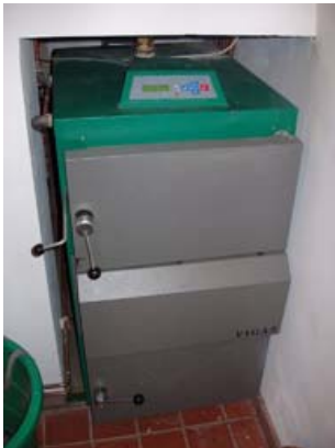
Vigas boiler under stairs at home in Washford
